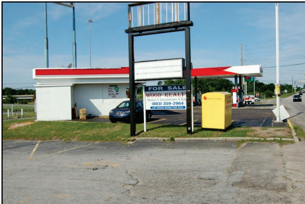
Figure 5.35: Resource 106-6395 (830 Bush River Road) – View of the east side elevation, facing west.
