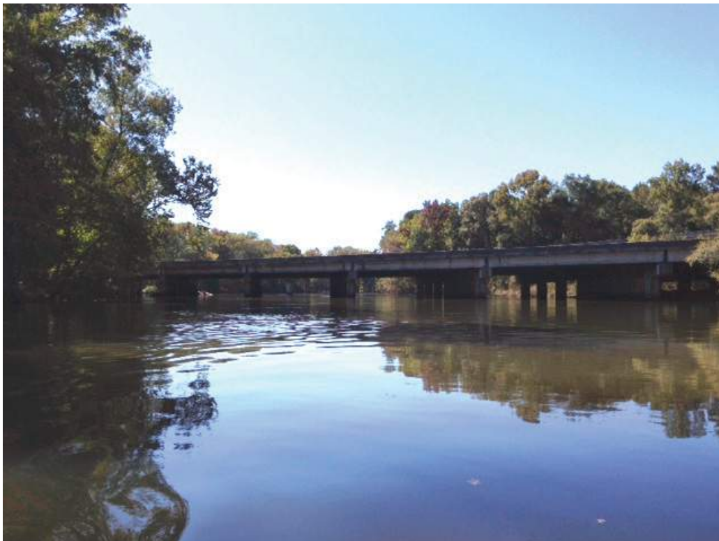
Photograph 6. View facing west at the Interstate 26 bridge crossing of the Saluda River.
