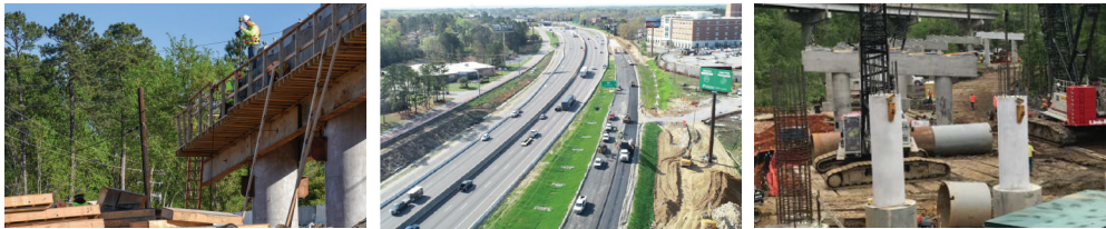
Picture 1: Bridge under construction near Colonial Life Blvd.; Picture 2: Construction of the ramp expansion along I-26 eastbound; Picture 3: Drilled shaft preparation for a bridge near the Saluda River.
