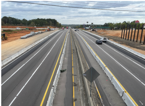
I-20 looking east. Various construction activities happening along I-20 eastbound and westbound.
