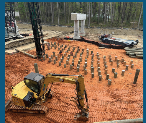
Timber pile stabilization near the Saluda River near I-26 westbound.
