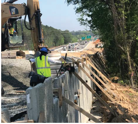
MSE wall being installed along McSwain Drive. An MSE wall is a type of retaining wall.
