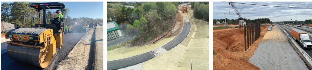
Picture 1: Asphalt paving of new collector distributor ramp on I-20 westbound; Picture 2: Construction of Garner Lane relocation; Picture 3: Pile foundation for southbound Broad River Road bridge over I-20.
