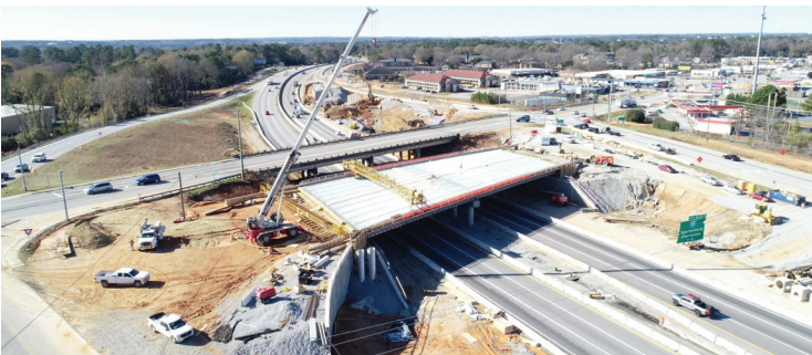
Overview of progress of the first of three bridges to be erected near Broad River Road.
