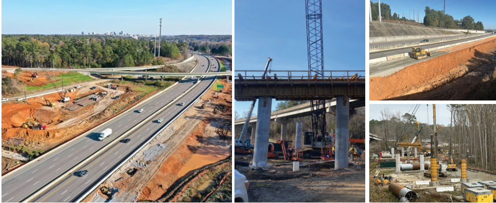
Images of construction in various stages for the Colonial Life Boulevard at I-126 Interchange
