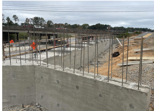
New Broad River Road bridge end cap that girders will be placed on.
