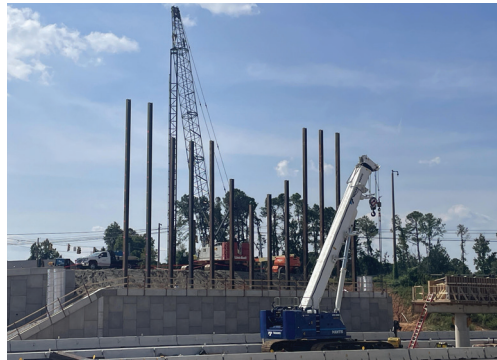
Nearly completed retaining wall for the new Broad River Road bridge currently under construction over I-20.
