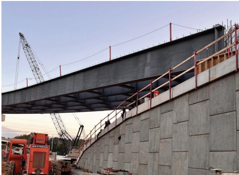
Steel girders and MSE wall for Ramp from Colonial Life Blvd to I-126 westbound.
