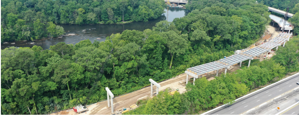
A new bridge over the Saluda River from I-26 westbound to I-126 eastbound being constructed.
