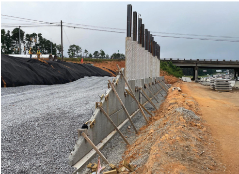
Bridge piles that will support the end of the new Broad River Road bridge. A new retaining wall is also being constructed.
