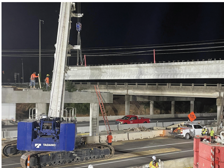
A concrete beam being set on a new Broad River Road bridge that will extend over I-20.
