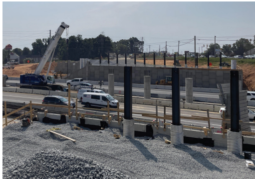
Bridge piles for both end bents as well as the center columns to support the new Broad River Road bridge over I-20.
