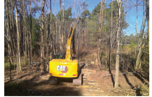
Tree clearing and logging is taking place in Phase 1 to prepare for bridge construction.
