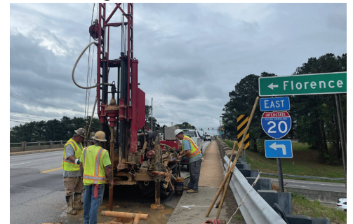
Soil boring samples provide data on the most appropriate, efficient, and sustainable foundation and roadbed design.
